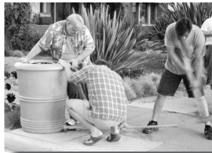
David Jirik, Martin Van Der Roest and Javier Garcia use teamwork and brute strength to install the 900 pound concrete receptacle on 10th Street.
